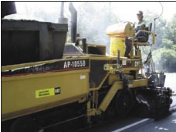
Asphalt is applied just moments after the GlasGrid® is laid in place with Caterpillar AP-1055B.
