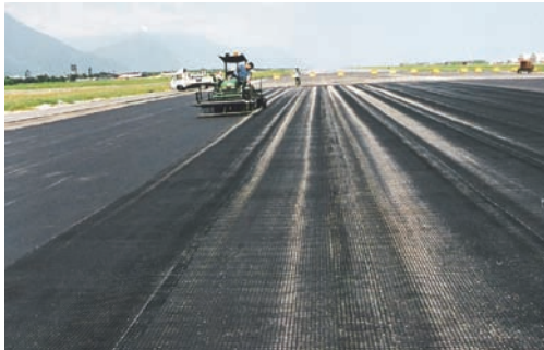
The GlasGrid System was installed over the entire length and width of the runway.
