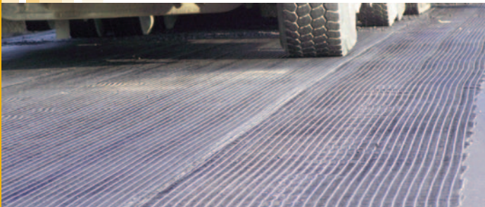
The GlasGrid® System is able to withstand construction equipment trafficking before being overlaid.
